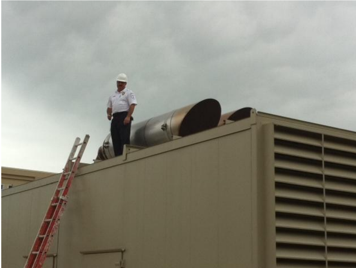
Frank Marshall inspects one of the two natural gas generators.
